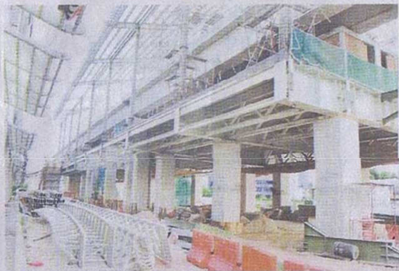
Sunway Construction would build and complete the viaduct guideway and other associated works for a 4.9km stretch of the SSP Line's elevated alignment from Sungai Buloh to Persiaran Dagang.
